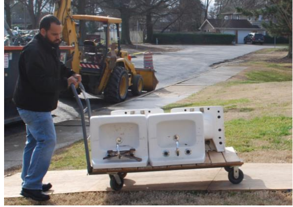
Sinks from the former Lake Taylor Health Center in Norfolk have been reused in the Brock Environmental Center.
