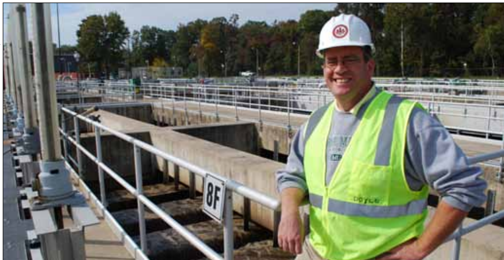
The Noman Cole sewage treatment plant in Lorton, Virginia, is one of the 21 being improved across the Commonwealth, requiring the hiring of thousands of workers. Fairfax County Senior Engineer Matthew Doyle is helping to supervise the project in Lorton.
