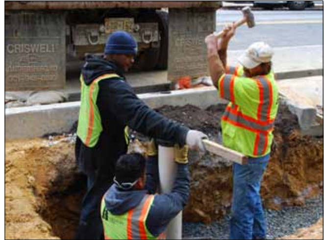
Workers build a stormwater pollution control device called a “bumpout” in Montgomery County, Maryland.
