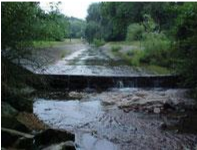
Before restoration, Spring Branch flowed through a concrete channel, and obstructed fish passage.
