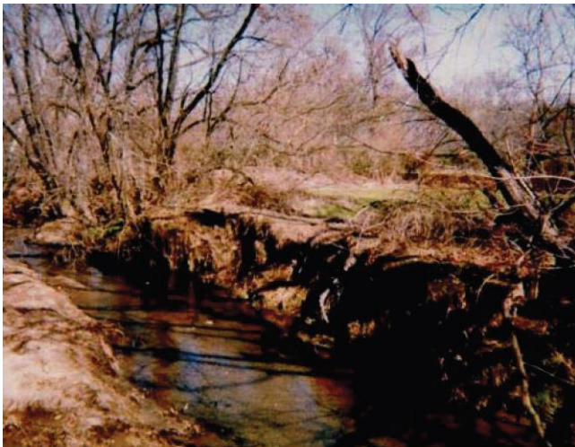
Mill Creek before restoration, 2004
