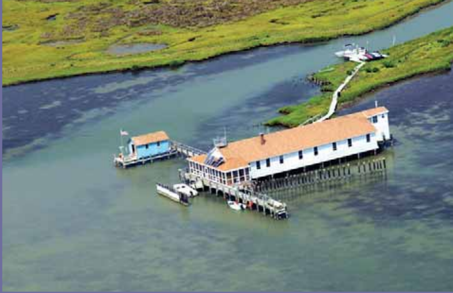
The Austin Memorial Foundation of Virginia made education programs at some of CBF's field programs possible with a first-time gift that funded roof repairs at CBF's Port Isobel and Fox Island (pictured above) Education Centers.
