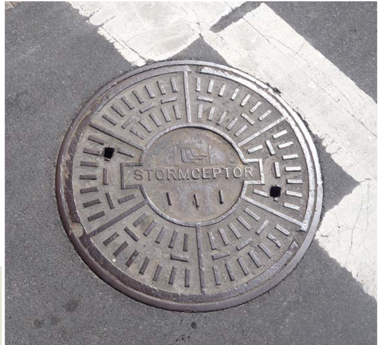
Stormceptor manhole cover
